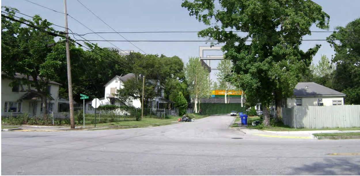
Facing east on Orvid Street from North Carolina Avenue with the Construction of the Earthen Berm.
